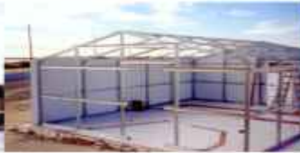
Girts and Purlin Hat Sections are installed every 5' for support of Paneling System.
