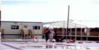
Two mechanics are able to install frames easily, all in one day.
